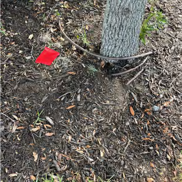
Zone #20 (Broken Drip or Micro Spray) - 06-08-26 8:51 am CDT
